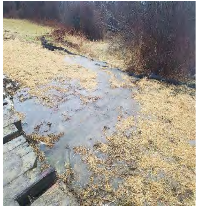
Fig 10: Filter sock needed fixing at wetland NW18 at Frink farm. Viewing north. (Corrections made.) (12-14-19).
