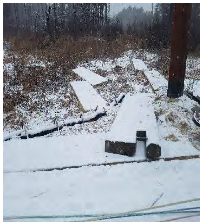
Fig 20: Filter sock installed around Str. 3. Excess mats are removed once line is pulled. Viewing west. (12-17-19).
