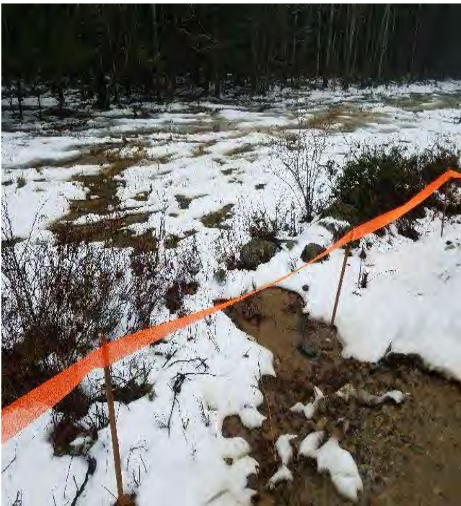
Fig 11: Sediment discharging into wetland DW2, recommend extending BMPs to this area. (Corrections made.) Viewing west. (12-14-19).
