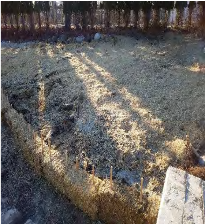
Fig 15: Soil pile at Str. 1 has been removed. Exposed soils mulched And BMPs installed downslope. Viewing southwest. (12-16-19).
