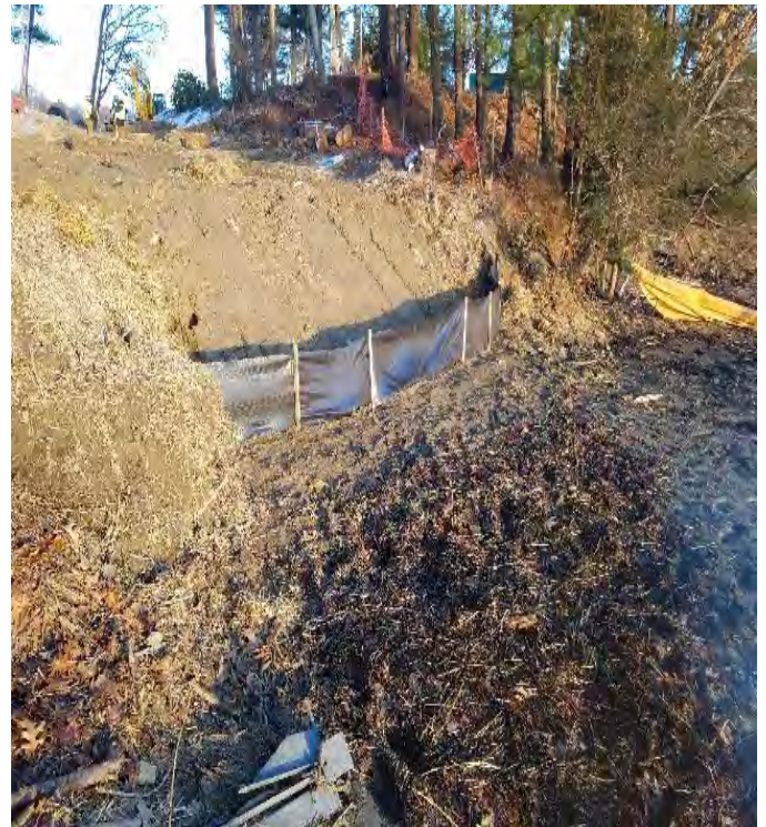
Fig 4: Restoration of slope at Gundalow landing/east side of the Bay. Viewing east. (12-12-19).
