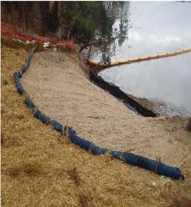
Fig 7: Crew installing sediment and erosion controls at Gundalow landing/east side of the Bay. Viewing south. (12-13-19).
