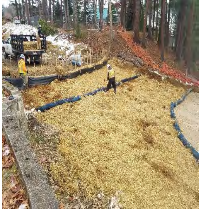
Fig 6: Crew installing sediment and erosion controls at Gundalow landing/east side of the Bay. Viewing east. (12-13-19).
