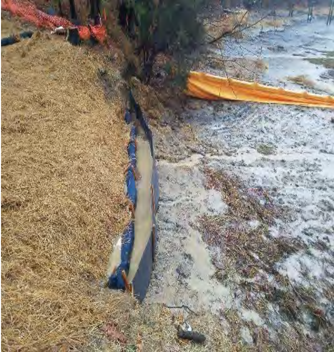
Fig 9: Sediment build up behind silt fence at Gundalow landing/east side of the Bay. (Corrections made.) Viewing south. (12-14-19).
