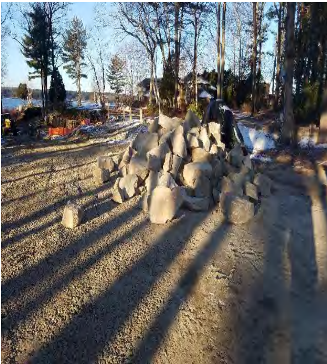
Fig 3: Large diameter stone used for restoring the slope at Gundalow landing/east side of the Bay. Viewing west. (12-12-19).
