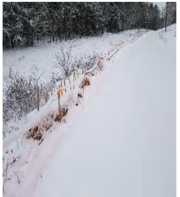
Fig 24: Crew extended row of BMPs along access road to Str. 99. Viewing west. (12-18-19).
