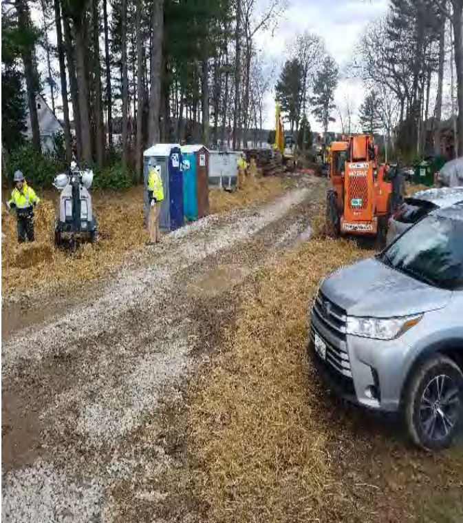
Fig 13: Crew spreading straw over exposed soils at Gundalow landing/ east side of the Bay. Viewing west. (12-15-19).
