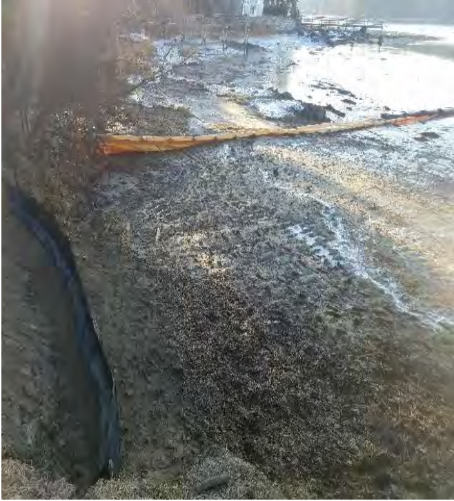
Fig 5: Silt curtain and BMPs installed at Gundalow landing/east side of the Bay. Viewing south. (12-13-19).
